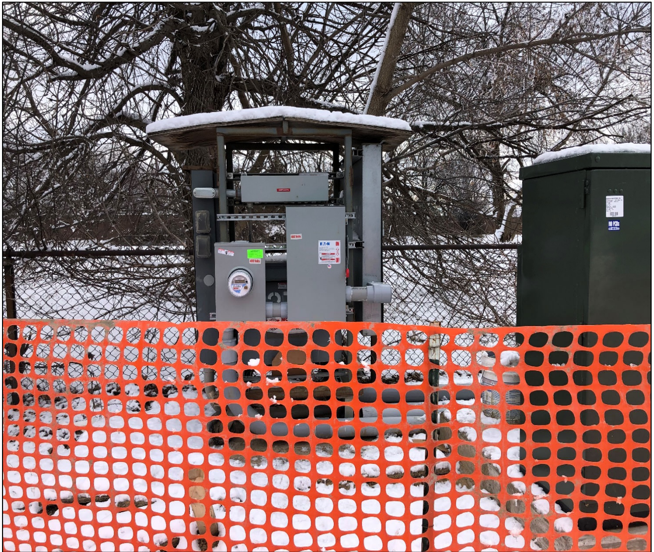
Figure 7 – Temporary Power w/DTE Meter
