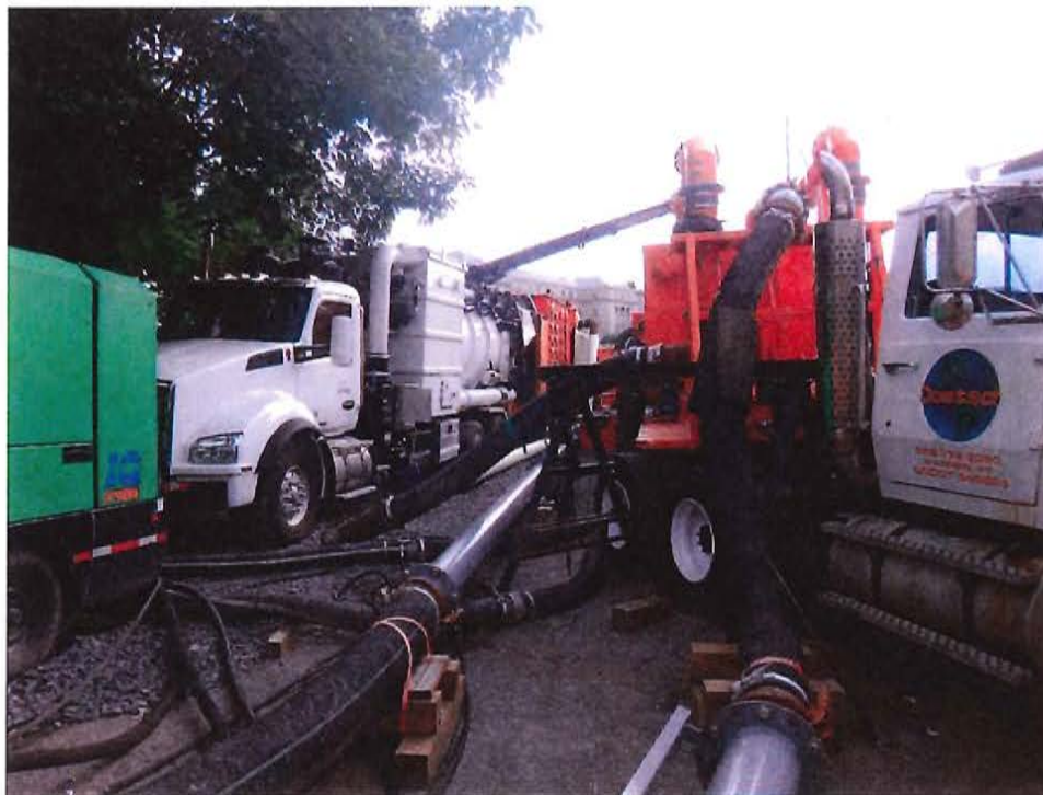
Debris / water separator, air compressor and vacuum truck. Outside building.
