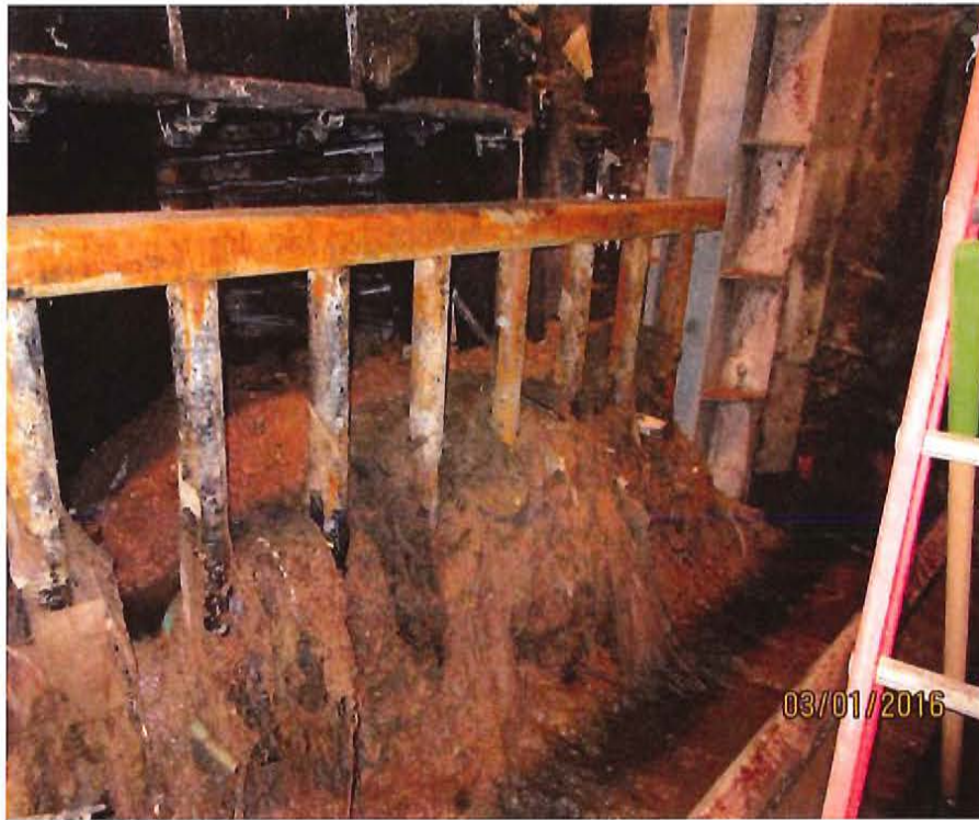
Impact rack used at DC Potomac Pump Station
