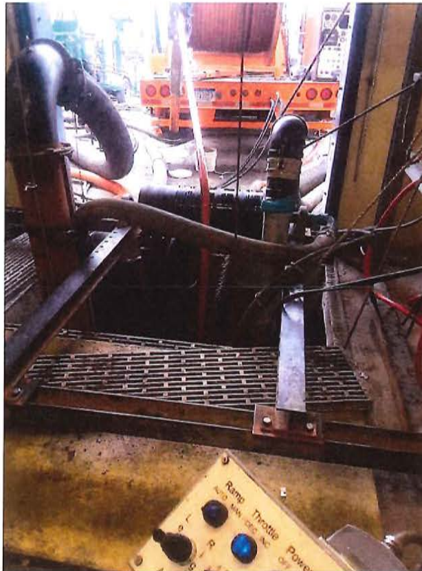
Inside the pump station looking out
