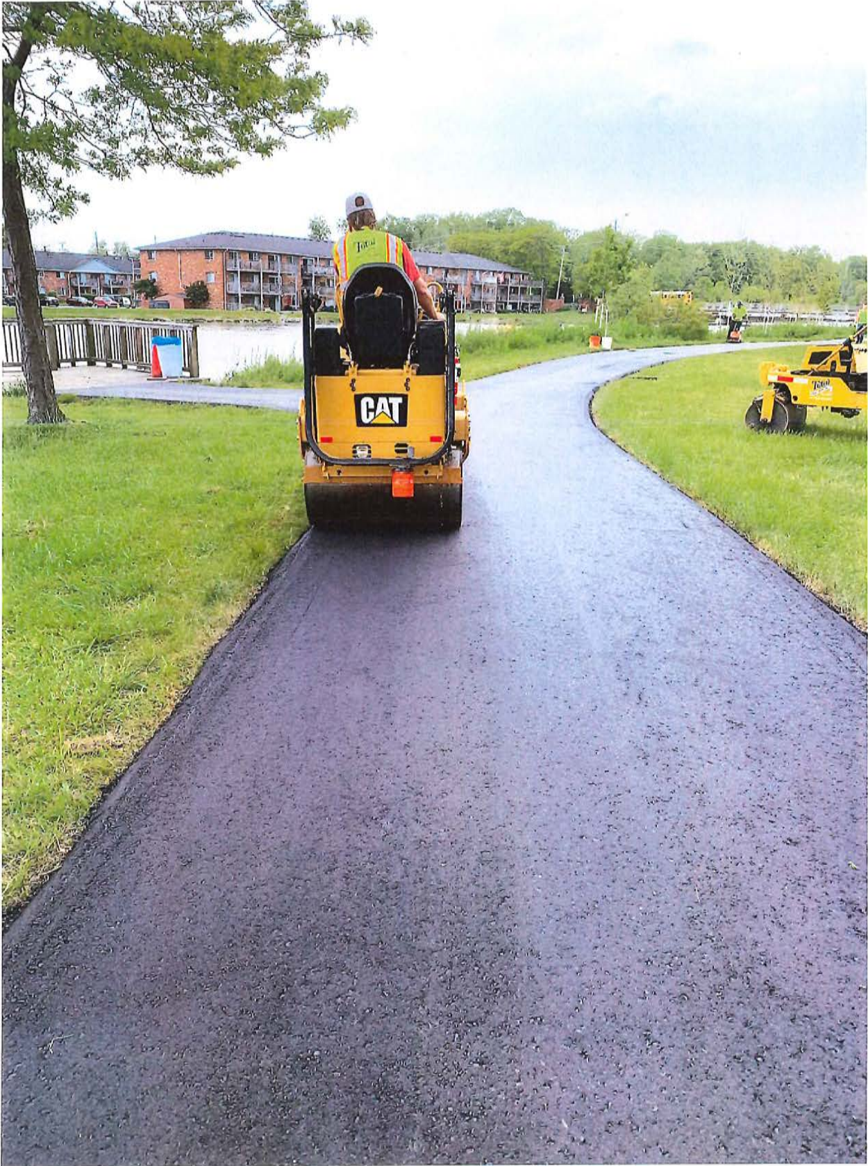
Jefferson Spillway Park restoration 2" Asphalt cap on bike path add stone and grade parking area and site with layer of topsoil then Hydro-seeded
