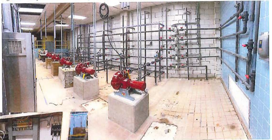
Figure 2 – Completed demolition, new plumbing, and system startup in Chapaton East Building Pump Room
