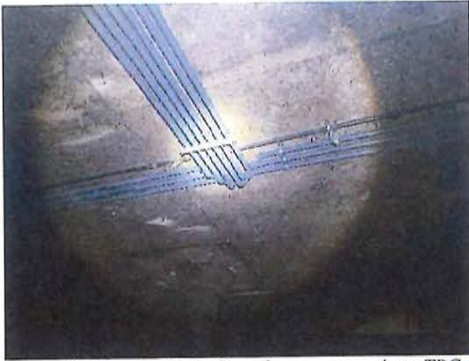
Figure 1 – Sample piping lines from pump racks to TRC units
