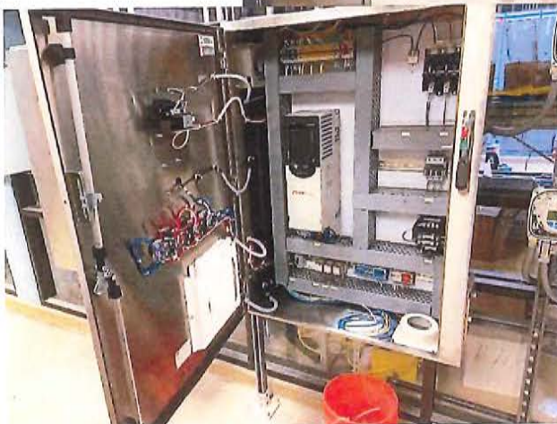
Figure 3 – New wiring and controls for hose pumps
